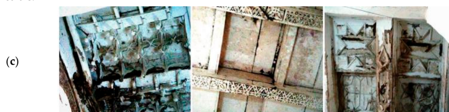
The gradual deterioration of the mihrab and dome, highlighting the loss of intricate details and vibrant colors.
